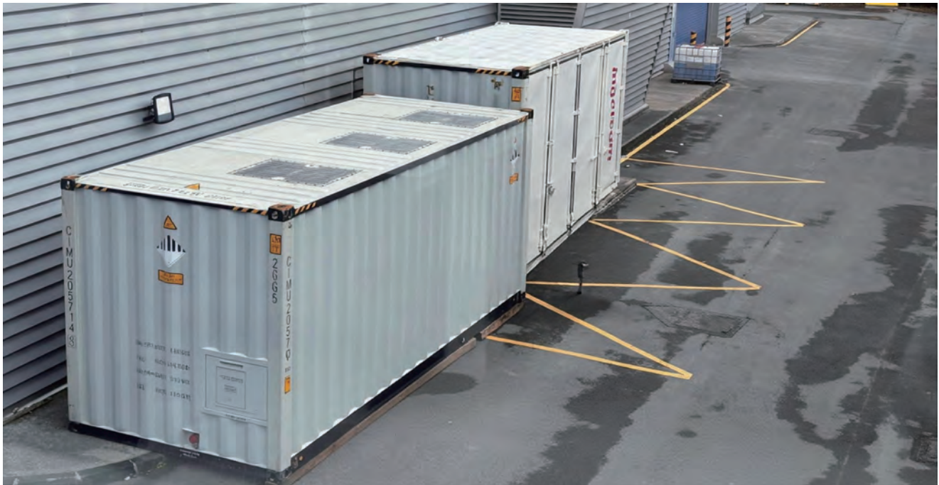
Figure: Sunwoda battery system undergoing integration testing at a well-known European PCS manufacturer's facility.
