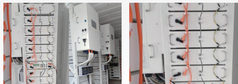
South Africa OASIS Flex & Deye 100kW/180kWh Battery System BESS for Resort
