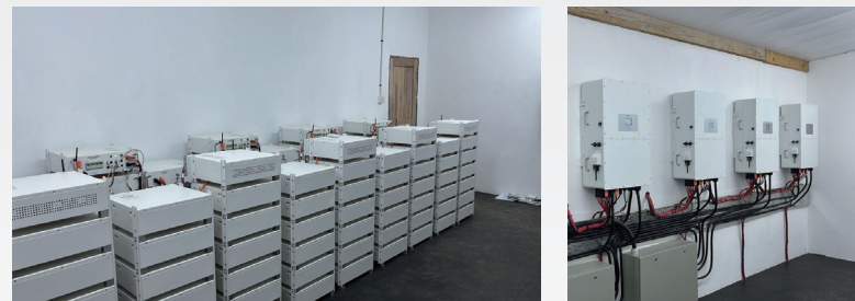
Zimbabwe OASIS Flex & Deye 250kW/600kWh Battery System BESS for Commercial Building
